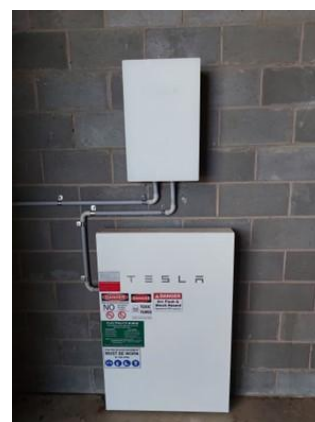
Figure 5: Solar battery installed at the Red Cliffs Depot.
