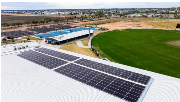
Figure 4: Solar installed at the Mildura Sporting Precinct.
