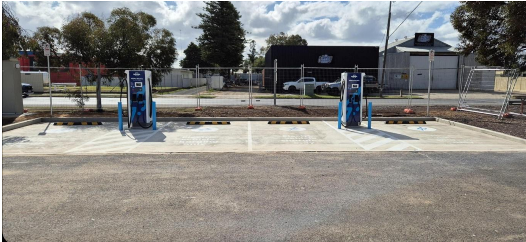
Figure 9: Electric vehicle charging stations in Hughes Street, Ouyen.
